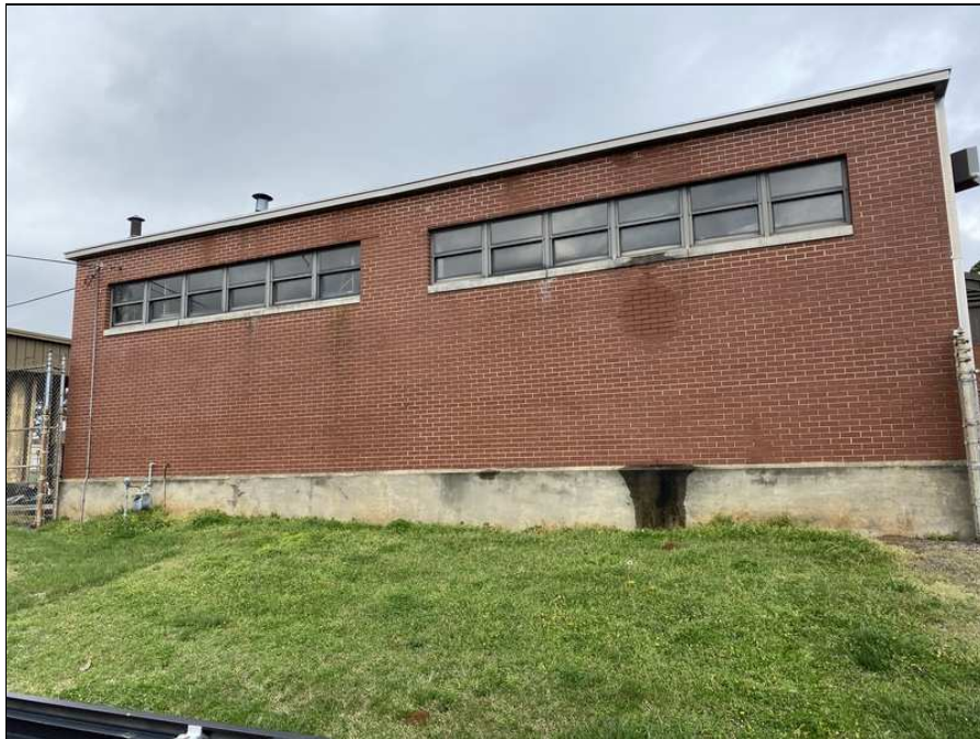
4 - View of the office building and non-ACM window caulking and rubber/silicone glazing.
